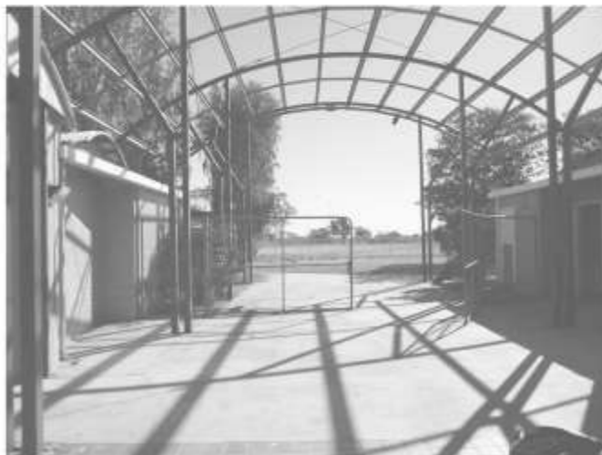
ENTRYWAY LATTICE TO BE REMOVED
